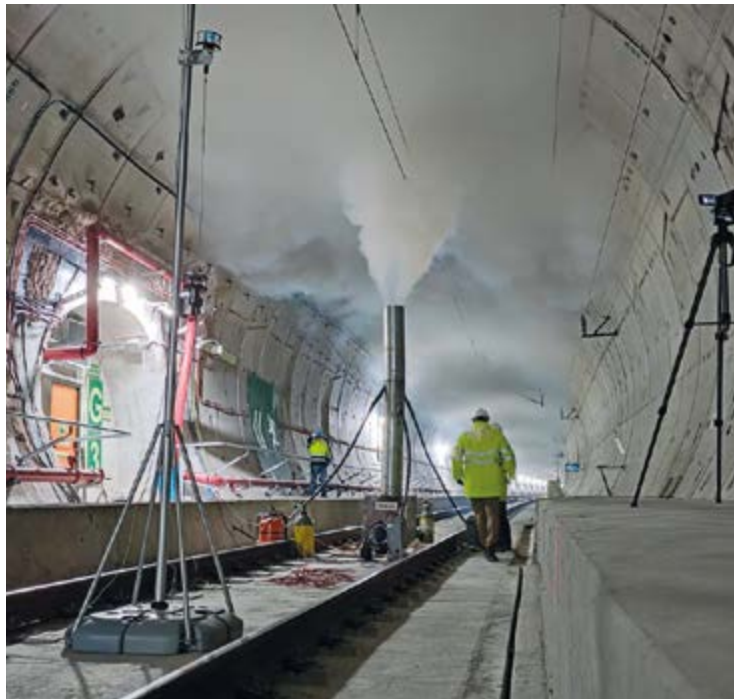
Civil protection and safety systems in the tunnels of the Pajares Bypass (Spain)
