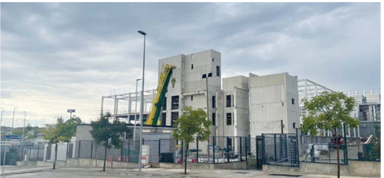
Data Centre for Equinix in Alcobendas, Madrid (Spain)
