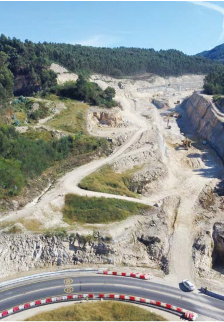
Stretch Vilaboa – A Ermida of the future Dual Carriageway A-57, Pontevedra (Spain)
