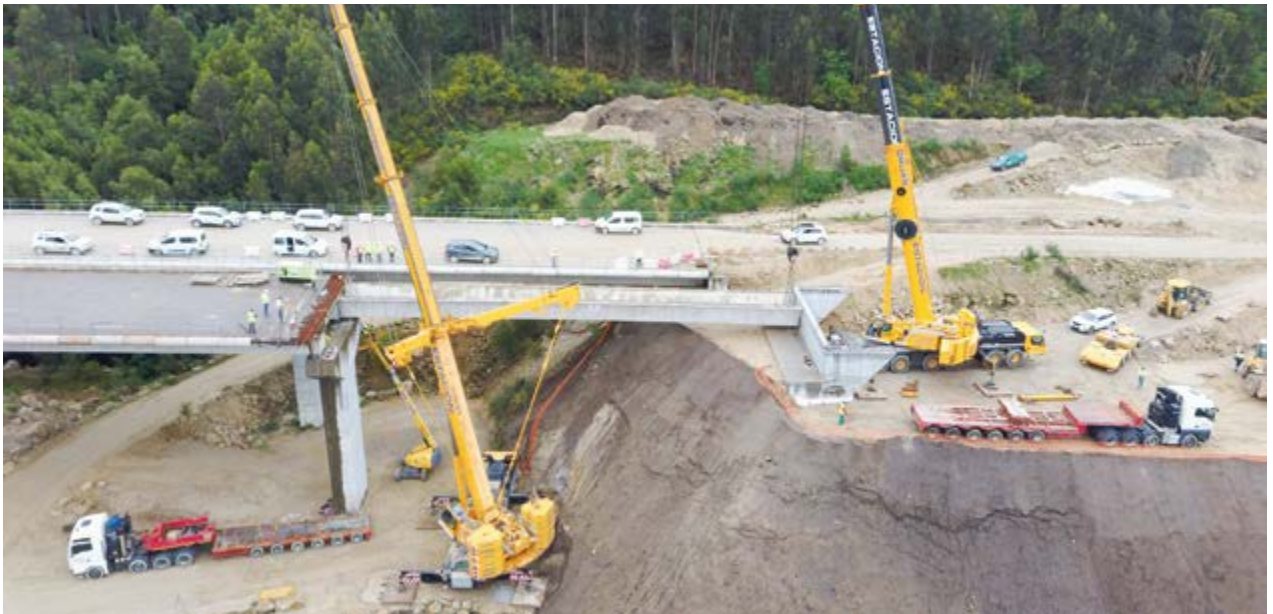
Stretch Vilboa – A Ermida of the future Dual Carriageway A-57, Pontevedra (Spain)
